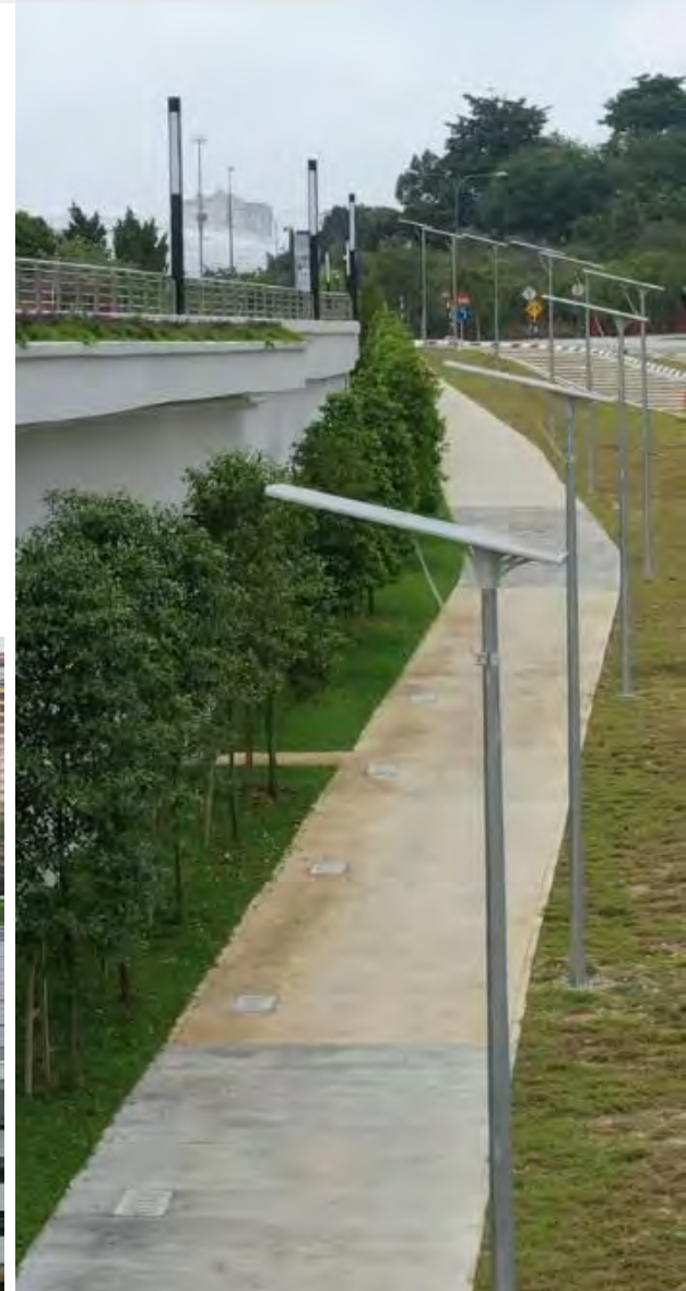
PV Street Lights-Bukit Jalil
