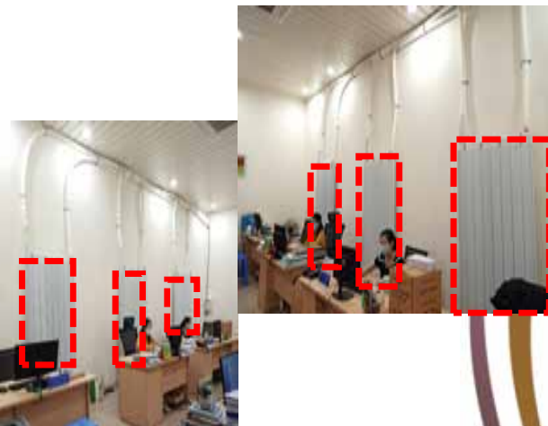
Radiant air conditioning system
