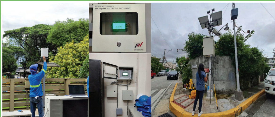
Images: Automatic Rain Gauges Water Level Sensor Seismic Accelerograph Source: Makati DRRMO
