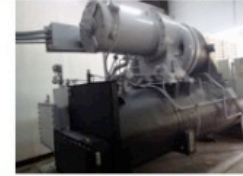
High efficiency air- conditioning and process cooling
