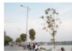
LED street lighting system
