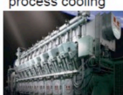
Co-generation system at factory
