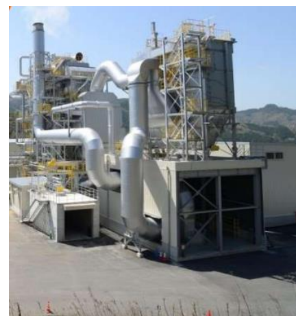
Biomass Power Plant
