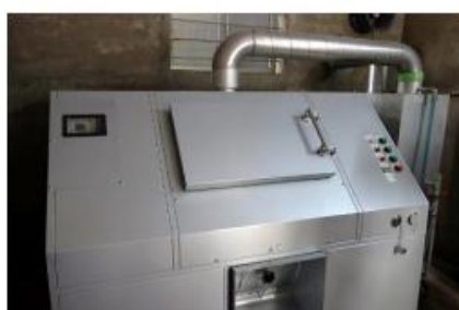
Composting Plant Installed
