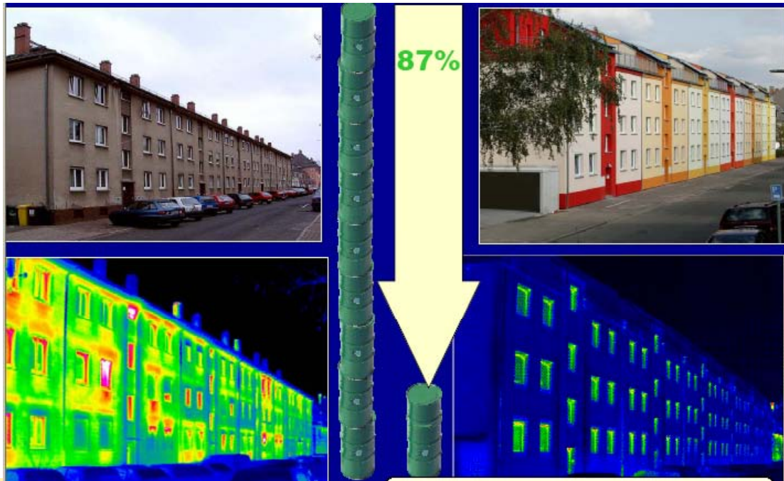
Above: photos Below: thermograms
