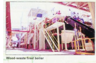
Wood-waste fired boiler
