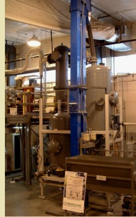
5 tpd biomass gasifier at BECON facility in Nevada, IA
